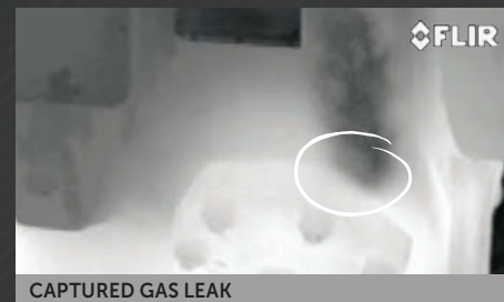
CAPTURED GAS LEAK
