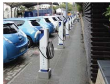
EV Charging Station
