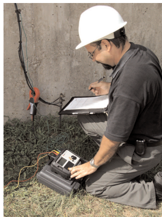
Using ART method with the DET3TC to test commercial ground without disconnecting the system
