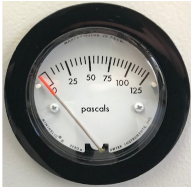
Figure 23: Analog pressure display (manometer) for monitoring the compressed air flushing on the chamber front
