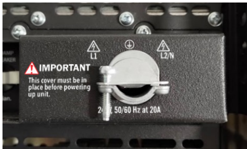
Figure 3.8 – AC Inlet Safety Cover
