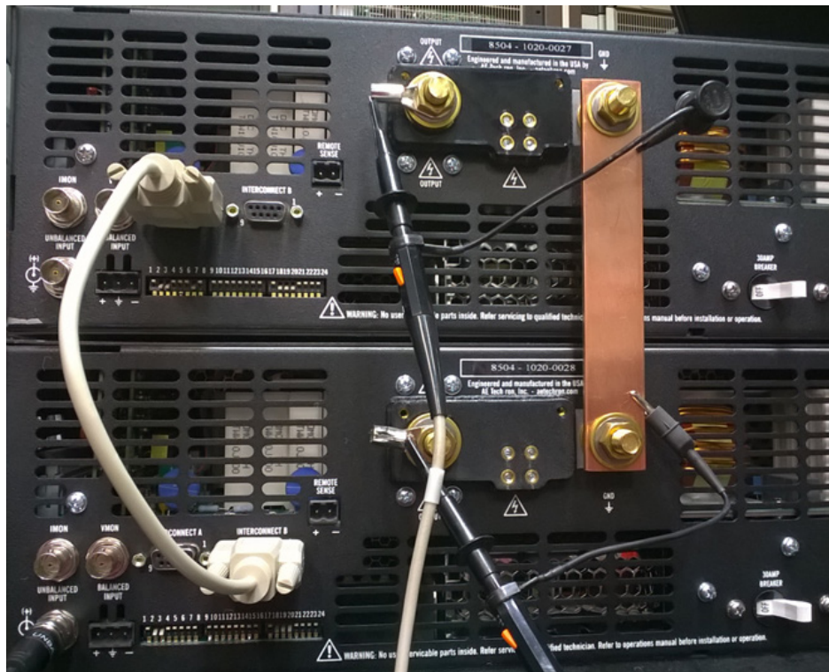
Figure 6.8 – Connecting the two amplifiers for parallel system testing
