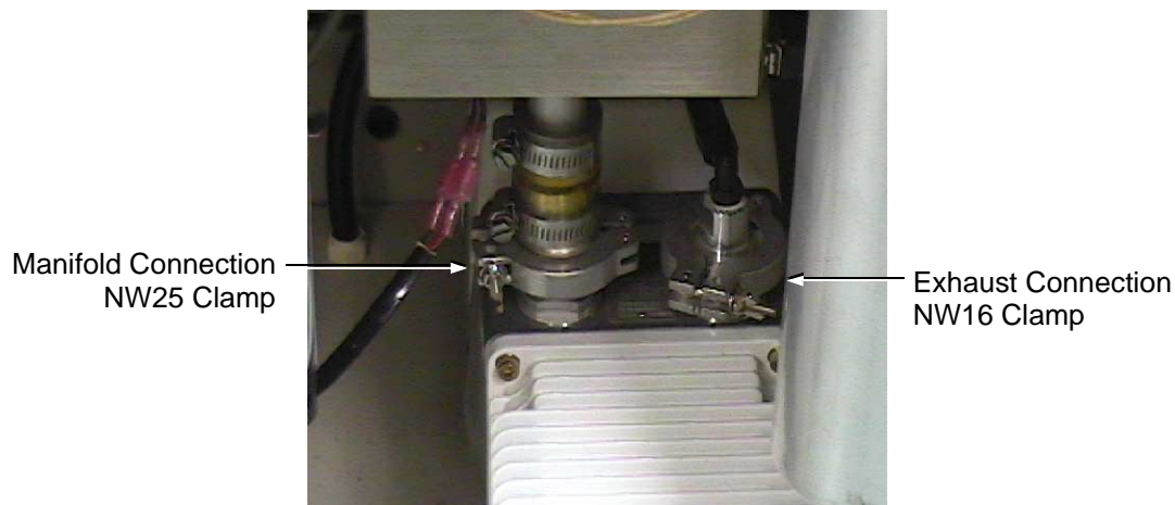
Figure B-11 Rough Pump Manifold and Exhaust Connections
