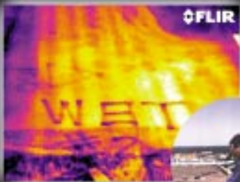
Wet insulation on a flat roof
