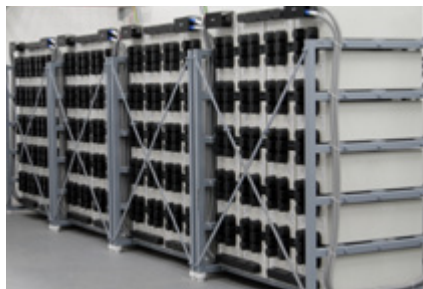
Energy Storage System
