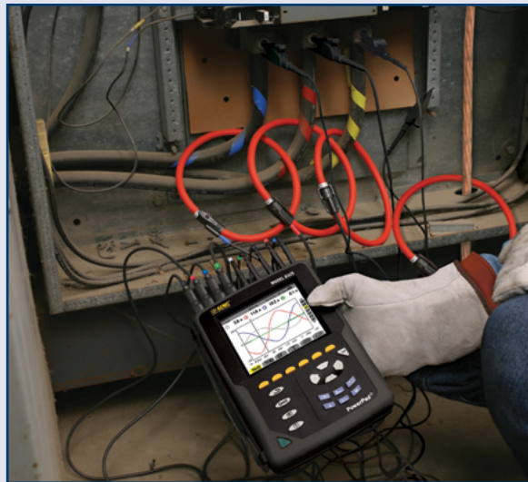
Power quality analysis on a three-phase panel using the AmpFlex ® flexible current probes.
