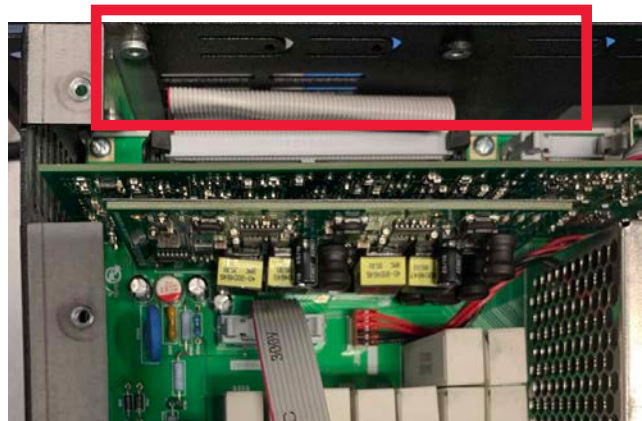
Figure 5.6 – Front-end board location
