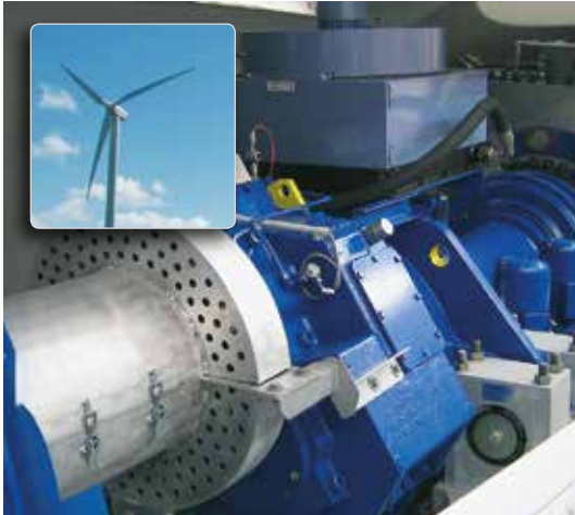
Easy-Laser® is used to align generators and gearboxes in wind turbines of a number of sizes and makes. Special brackets are available (accessories) for alignment with locked rotors, which increases the safety for the operator.
