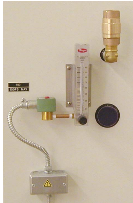
GN2 Purge System
