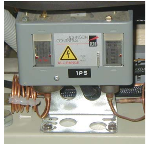
High / Low Pressure Switch
