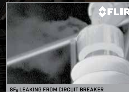
\text{SF}_6 LEAKING FROM CIRCUIT BREAKER
