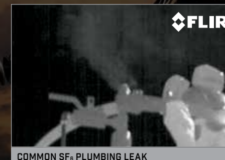
COMMON \text{SF}_6 PLUMBING LEAK
