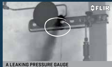
A LEAKING PRESSURE GAUGE
