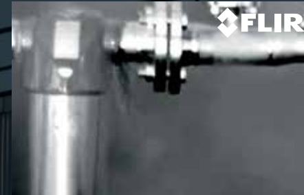
SPOT HARD-TO-FIND CO 2 LEAKS
