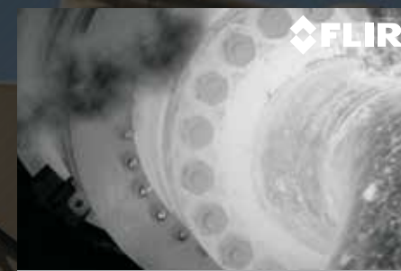
NATURAL GAS LEAK ON COMPRESSOR VALVE
