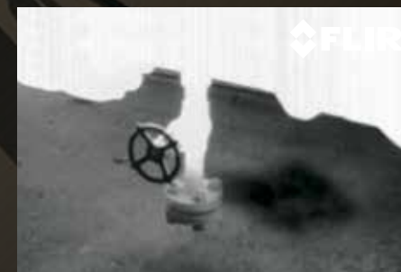
METHANE LEAK AT NATURAL GAS FACILITY SITE
