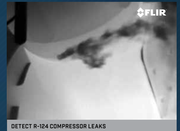
DETECT R-124 COMPRESSOR LEAKS
