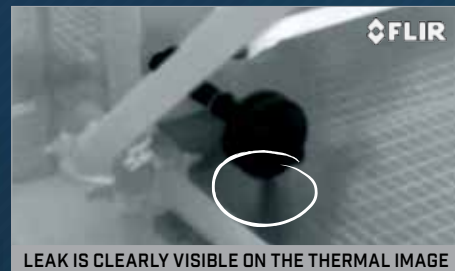
LEAK IS CLEARLY VISIBLE ON THE THERMAL IMAGE
